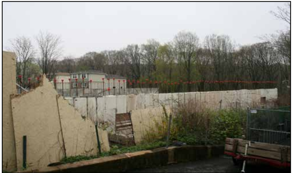
A side view of the construction, with houses on Clove Court in the background
